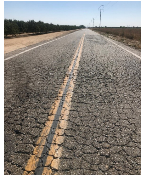
Alligator Cracking on Avenue 26 near Road 19
